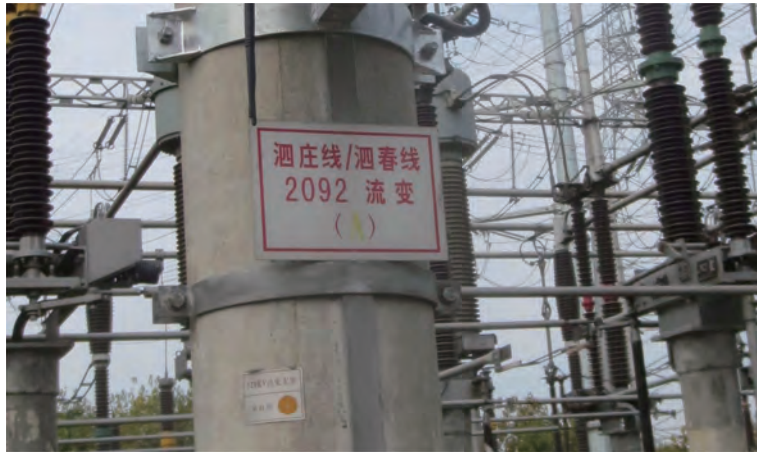
Figure 3.4: Tags of pillar in substation
