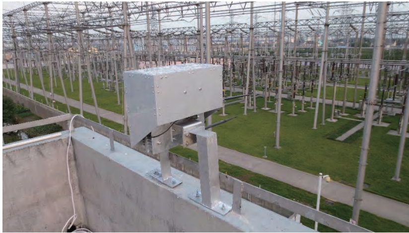
Figure 2.12: Substation of Sijing in Shanghai
